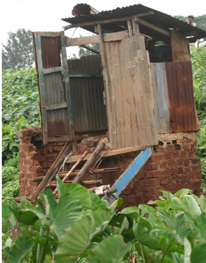
Figure 1: One of the Latrines Used by Patients
